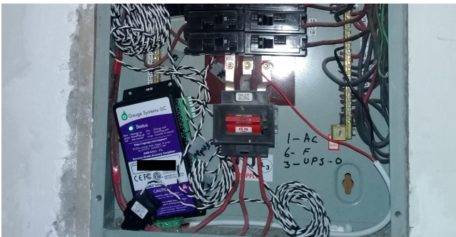
Figure 3: Smart meter installed in one of the selected households
